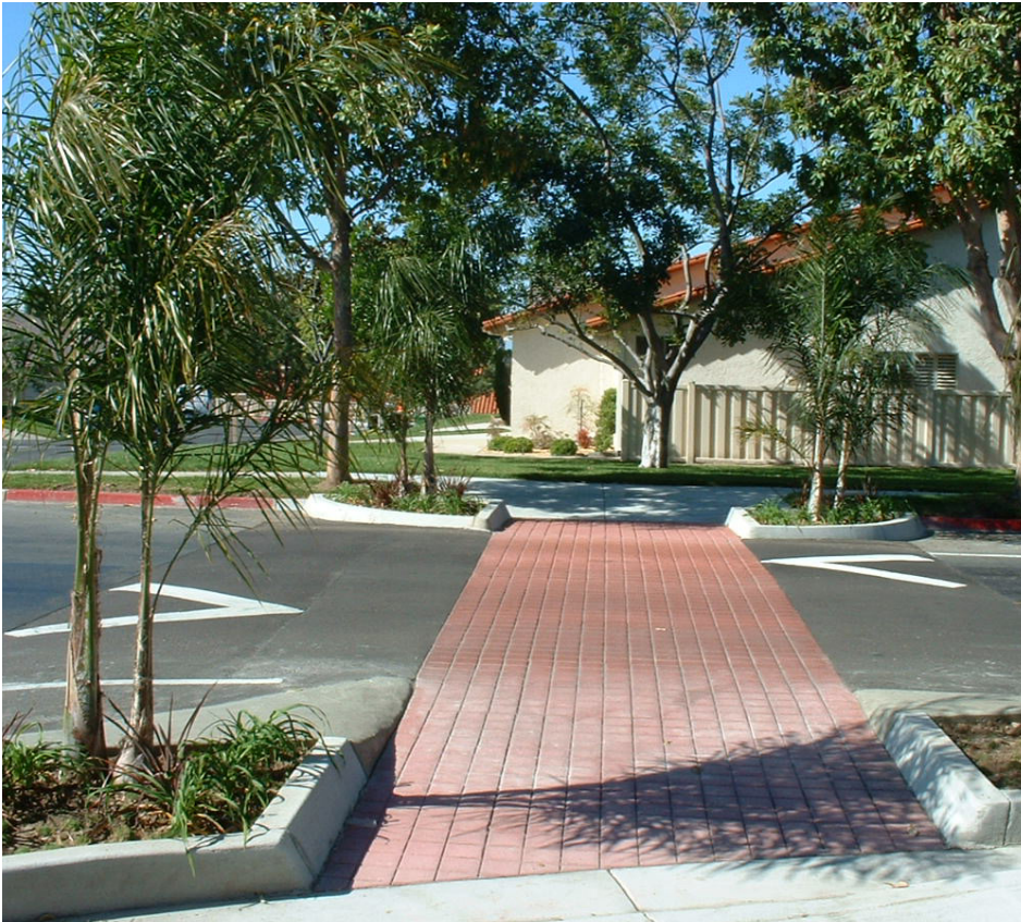
A raised crosswalk with bulb-outs. Source: Streetswiki.
