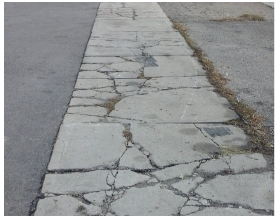
Significant sidewalk cracks on S. Federal Blvd.
