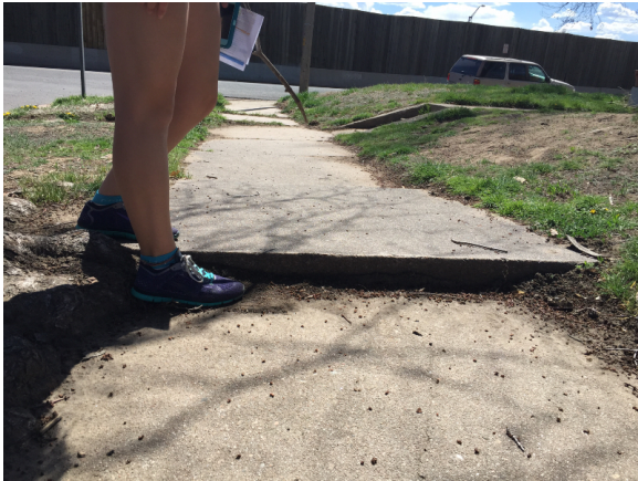
Uneven sidewalk on Irving Street between 48 th and 49 th Avenues
